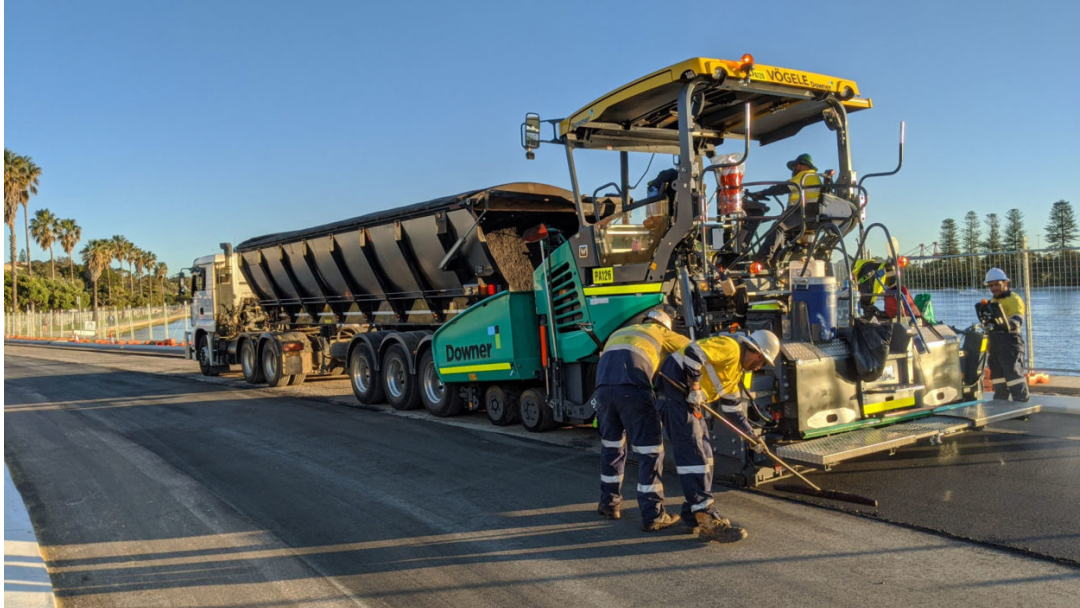
Asphalt with the additive TonerPlas, made from mixed soft plastics, is used to resurface a roadway in Fremantle, Western Australia, in 2020. COURTESY OF CLOSE THE LOOP
