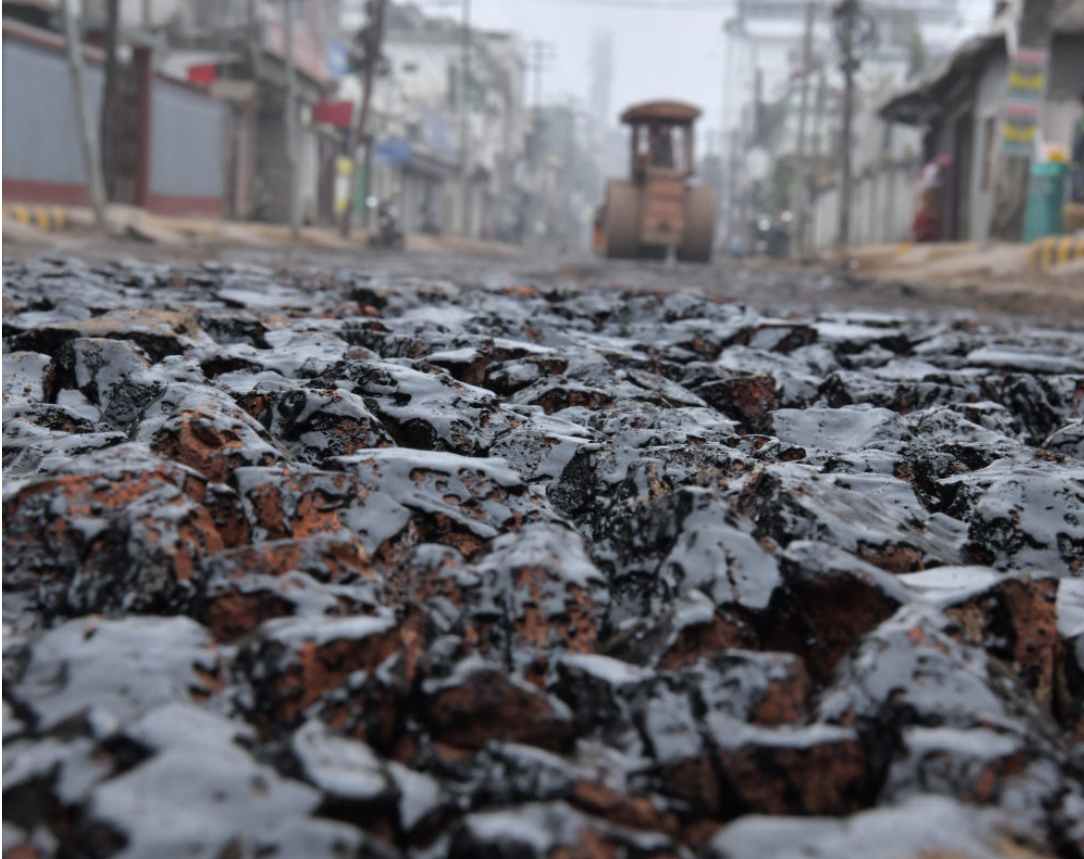
Workers lay down roadway made from plastic waste in Agartala, India, in January. XINHUA/STRINGER VIA GETTY IMAGES
