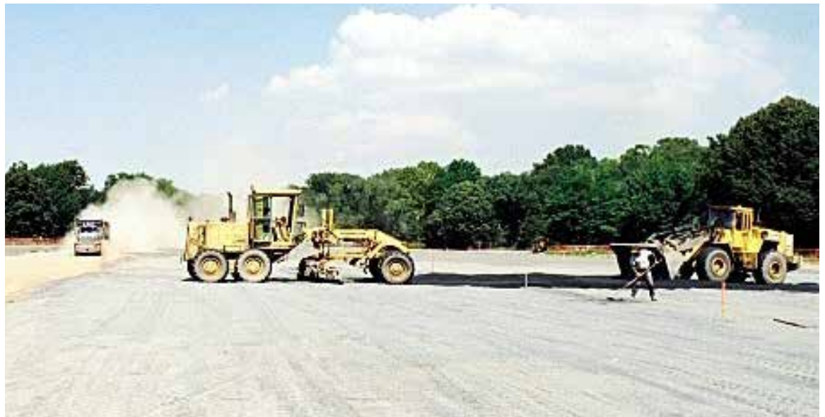
Figure 47. Spreading structural soil at Great Lawn in Central Park, New York, NY
