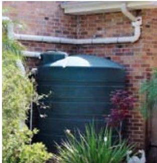
Cistern with plantings
