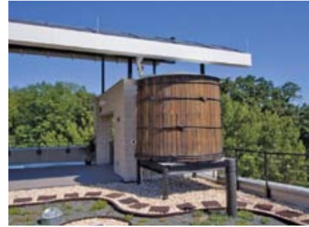
The appearance of rooftop cisterns can be softened with landscaping and careful choice of materials.
